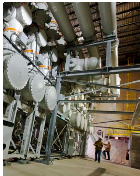
ComEd's West Loop station provides Chicago substations with multiple sources of energy supply – substantially reducing the likelihood of a significant loss of power downtown and in the surrounding Chicago neighborhoods.
