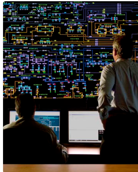
At PECO's Transmission Operations center in Philadelphia, operators keep close watch on the regional electric grid. PECO serves 1.6 million electric customers and 500,000 natural gas customers.
