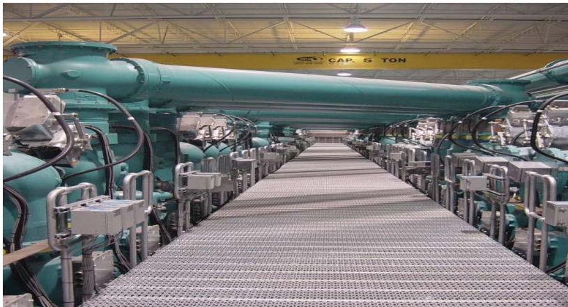
Inside Singer Substation
