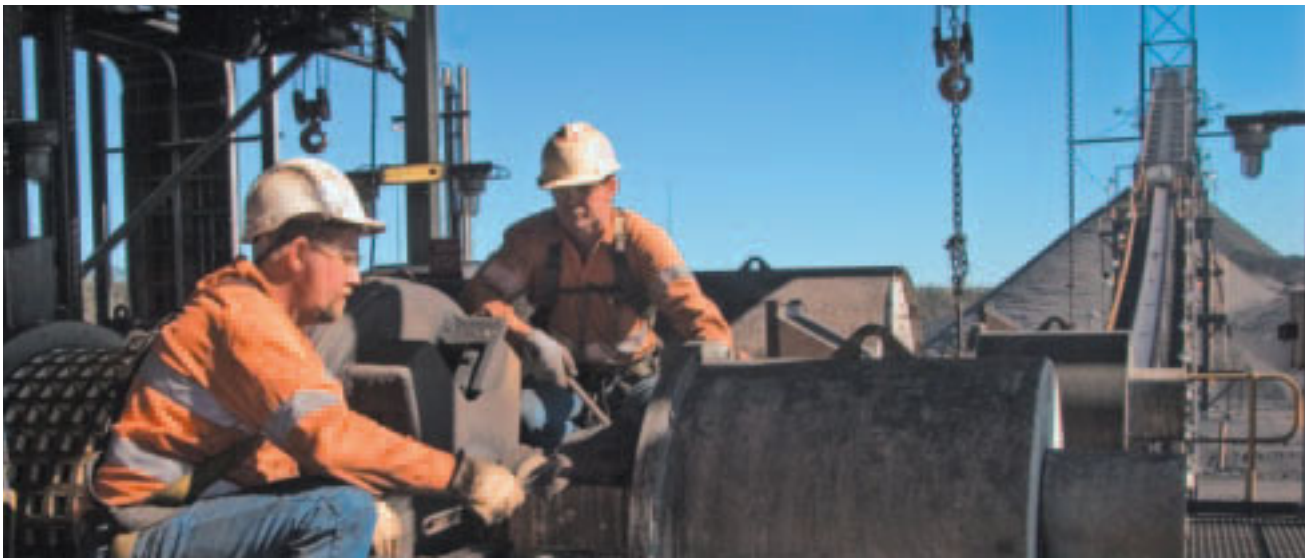
WAYNE CARUANA AND GREG WALES OF JSIS ENGINEERING PERFORMING MAINTENANCE WORK AT THE COPPABELLA MINE COAL HANDLING AND PREPARATION PLANT
