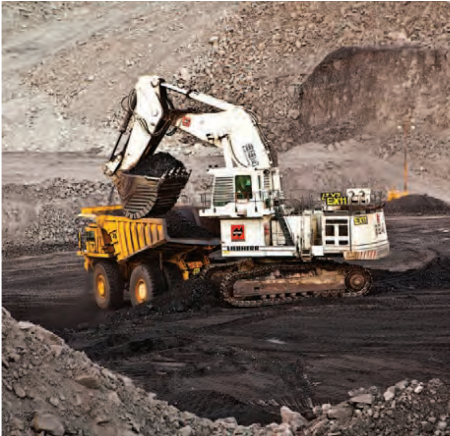
Excavator loading haul truck at Moorvale Mine – a total of 3.3Mt (100% basis) ROM coal was mined at Moorvale in FY2011.
