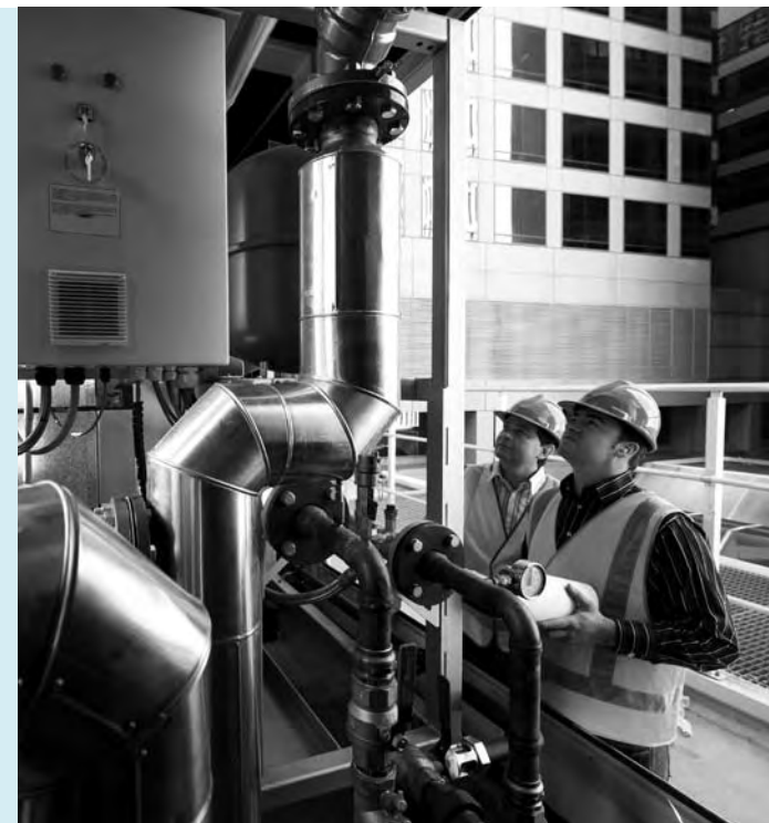
Tri-generation plant, Stockhome, NSW
