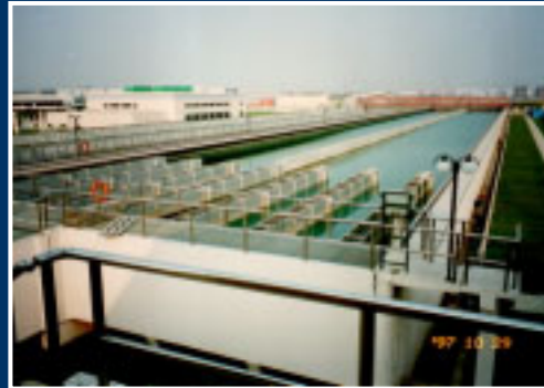
Dachang Water Plant, (BOT) GC
