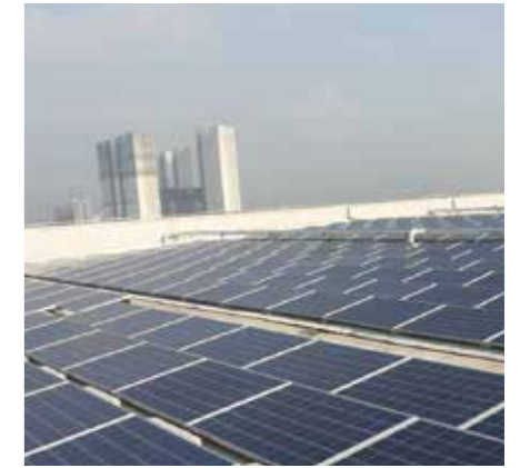
⬆️ Changzhou Youze Technology Factory Rooftop 680 KW Completion date: 2014/11
