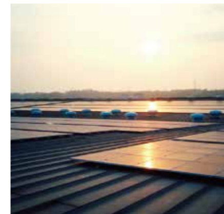
⬆️ Jiangsu Jintan Fanden Factory Rooftop 3860 KW Completion date: 2015/03
