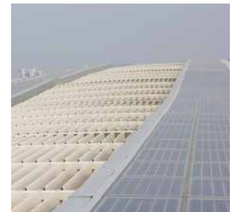
⬆️ Changzhou Train Station Rooftop 200 KW Completion date: 2011/05
