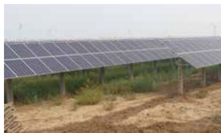
⬆️ Xiangshui project, Jiangsu Province, China 120 MW Completion date: 2014/12
