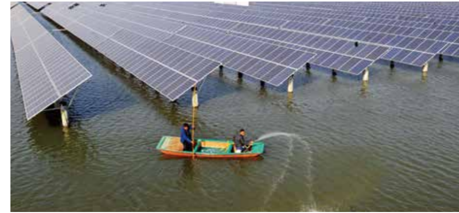
⬆️ Jiangsu Yanchen Fish Pond 1000 KW Completion date: 2014/12
