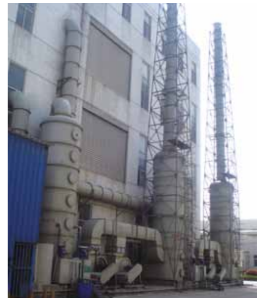
Scrubber of west campus
