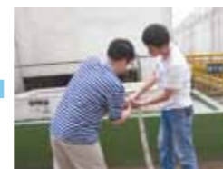
Water hose connection
