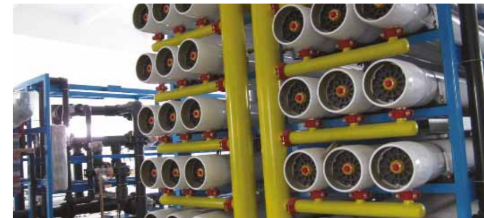
Ultra-filtration and reverse osmosis workshop
