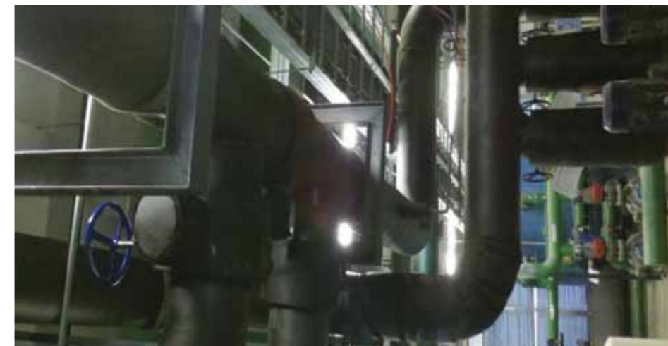
Plate exchanger for recycling residual heat
