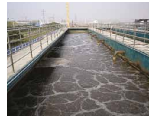
Upgraded waste water treatment facility
