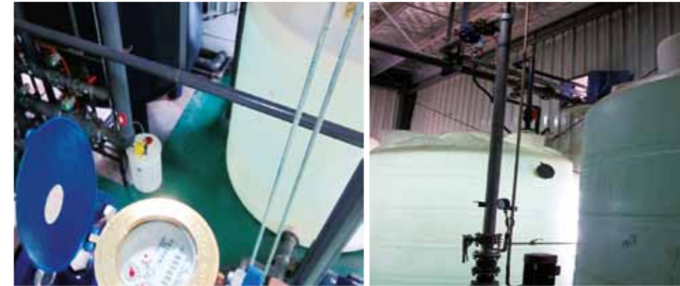
Water recycling equipment
