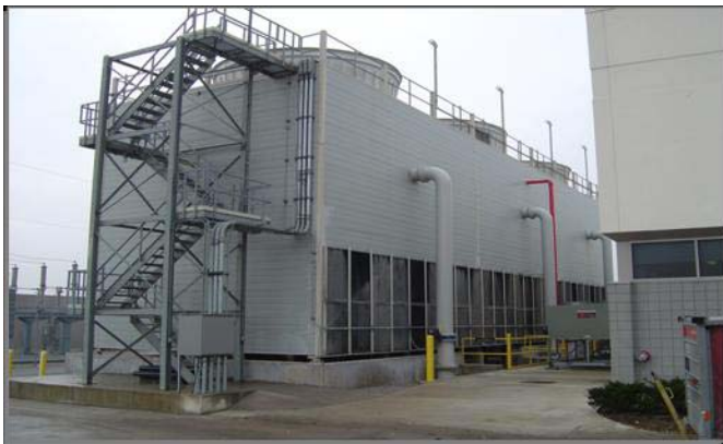
The Energy Center at McNamara Terminal Detroit, Michigan
