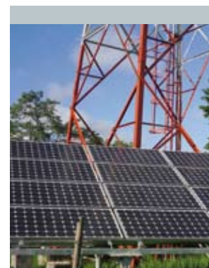
Solar panels powering our base stations in India
