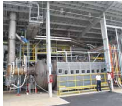
Air Products’ new combustion lab in Allentown, Pennsylvania, which serves customers in the glass, metals and energy industries.
