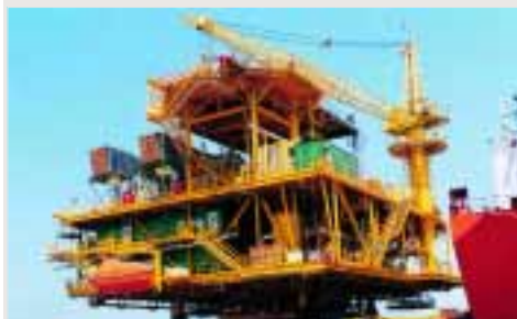
The OGGs platform topsides fabricated at the Stolt Offshore fabrication yard in Warri, Nigeria.
