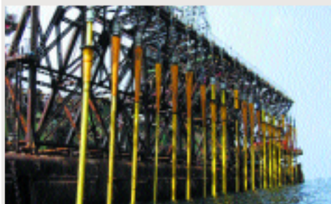
The Seaway Polaris holding production risers during an FPSO change out.
