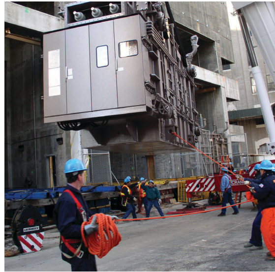
The reconstruction of the World Trade Center complex reached a milestone on November 8, 2003, when three electrical transformers were lifted into place at 7 World Trade Center.
