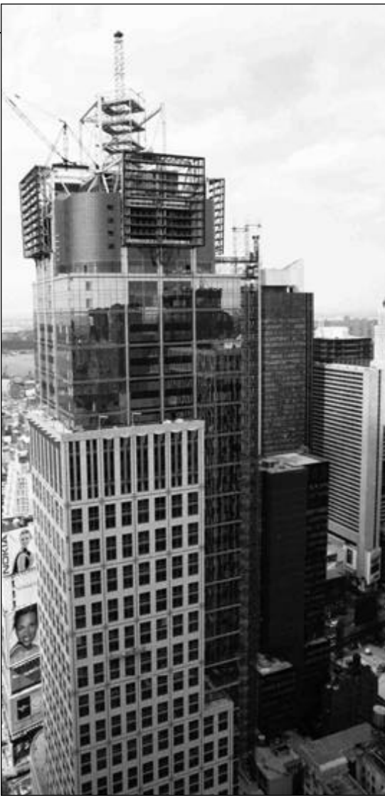
The New York City real estate market is booming, making building cranes a frequent skyline feature, as seen here in Times Square
