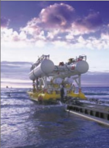
HALLIBURTON SUBSEA places a pre-fabricated offshore pipeline bundle with its Controlled Depth Tow Method.
