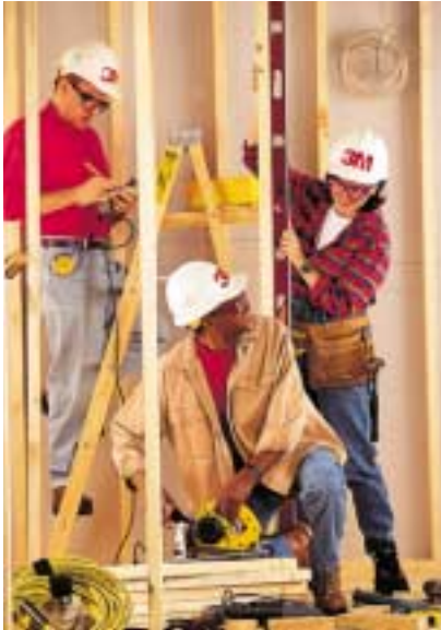
Habitat for Humanity volunteers from 3M help build and rehabilitate homes in the St. Paul metro area and other communities in the United States.
