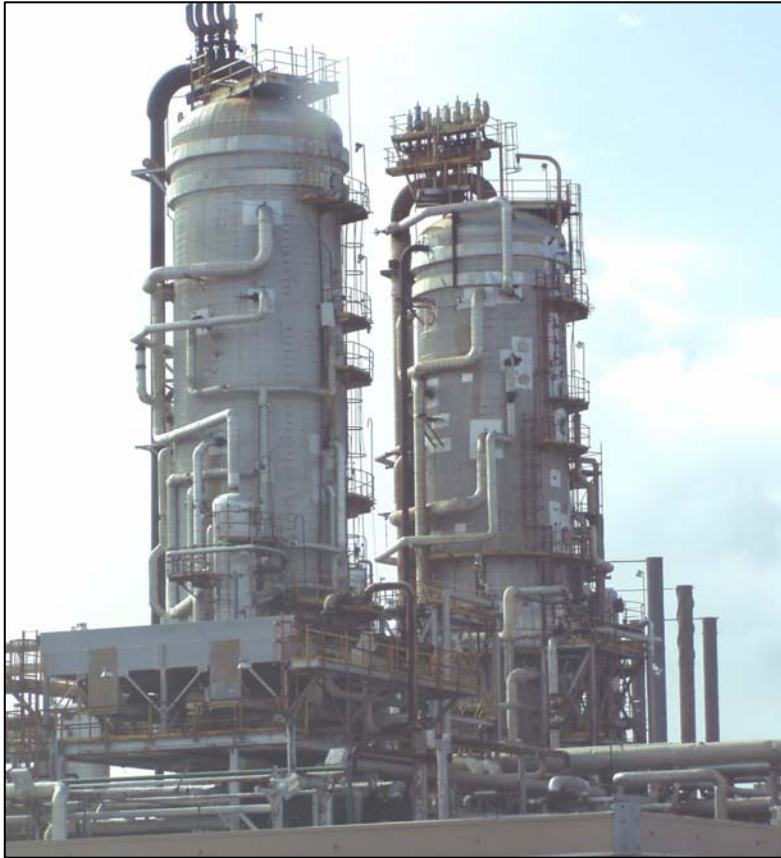
Aruba Crude Towers
