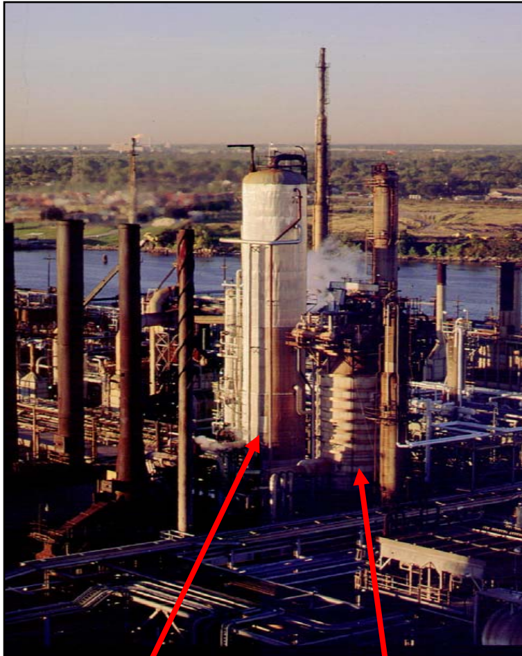
Crude Atmospheric Tower
