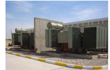
Electrical Transmission and Distribution Iraq
