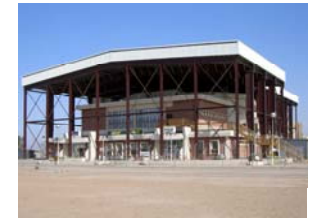
Overhead Coverage Systems (Iraq, Various Locations)
