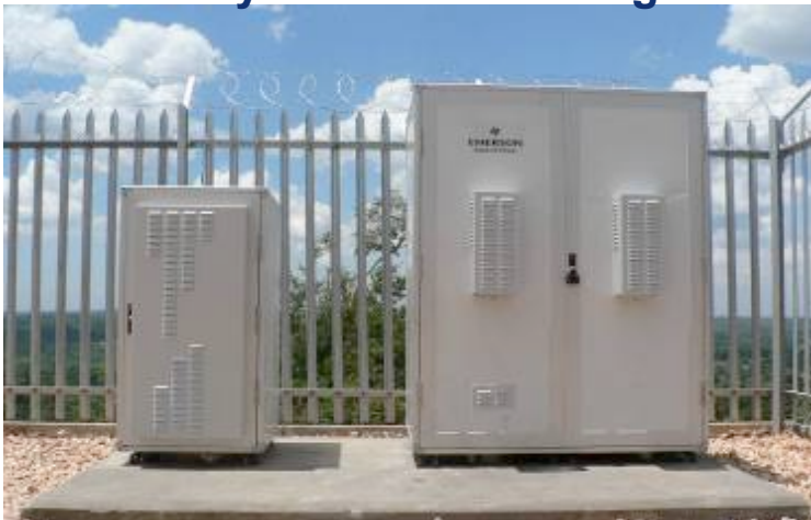
Power Enclosure Battery Enclosure
