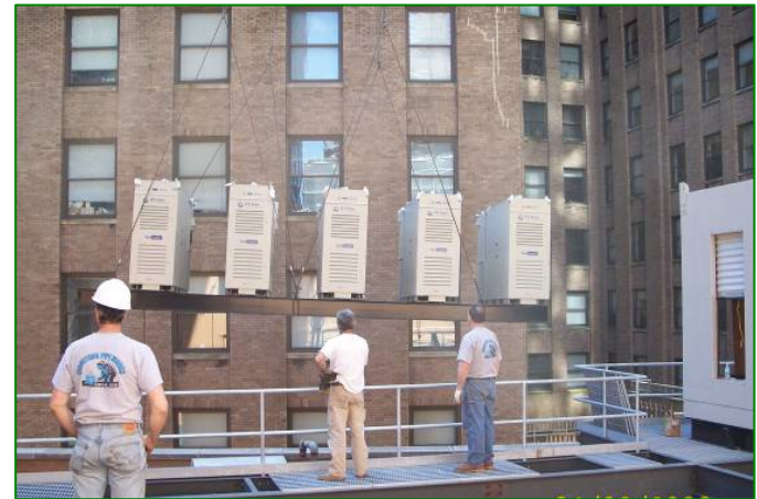
Installation at NY Downtown Marriott
