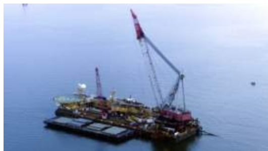
Natural Gas Pipeline Gulf of Mexico
