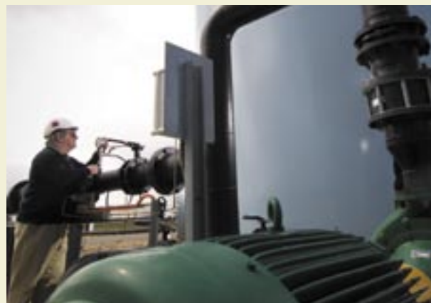
(Above) Ron Turnbull inspecting pipework and instrumentation which will receive high quality water from the Water Corporation's Kwinana Water Reclamation Plant.
