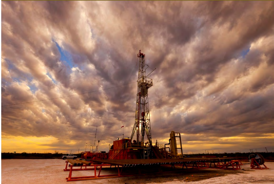
Drilling the Hutchins Stock Association #1096 in North Ward Estes Field, Whiting's EOR project in Winkler County, Texas.
