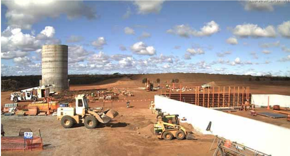
Figure 10: Concentrate plant site with ore bin on LHS, concentrate shed on RHS, footings for flotation plant and ROM pad in centre and back ground.
