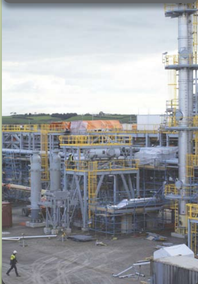
Pipe Rack at Kupe Production Station
