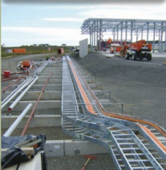
Pipe trays will carry 300km of cable around the Kupe Production Station
