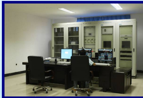
Compressed air control room
