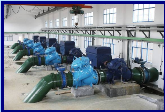
Cooling water pump station
