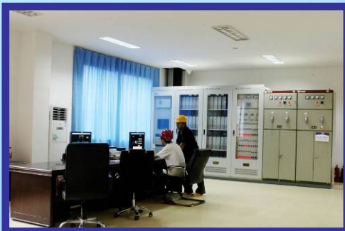
Switchgear control room
