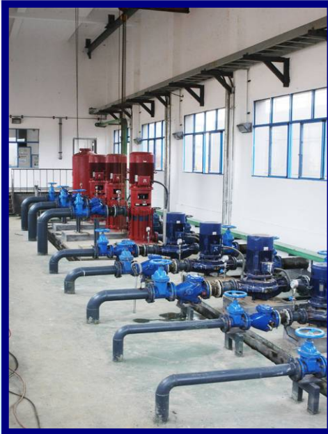
Fire water pump station
