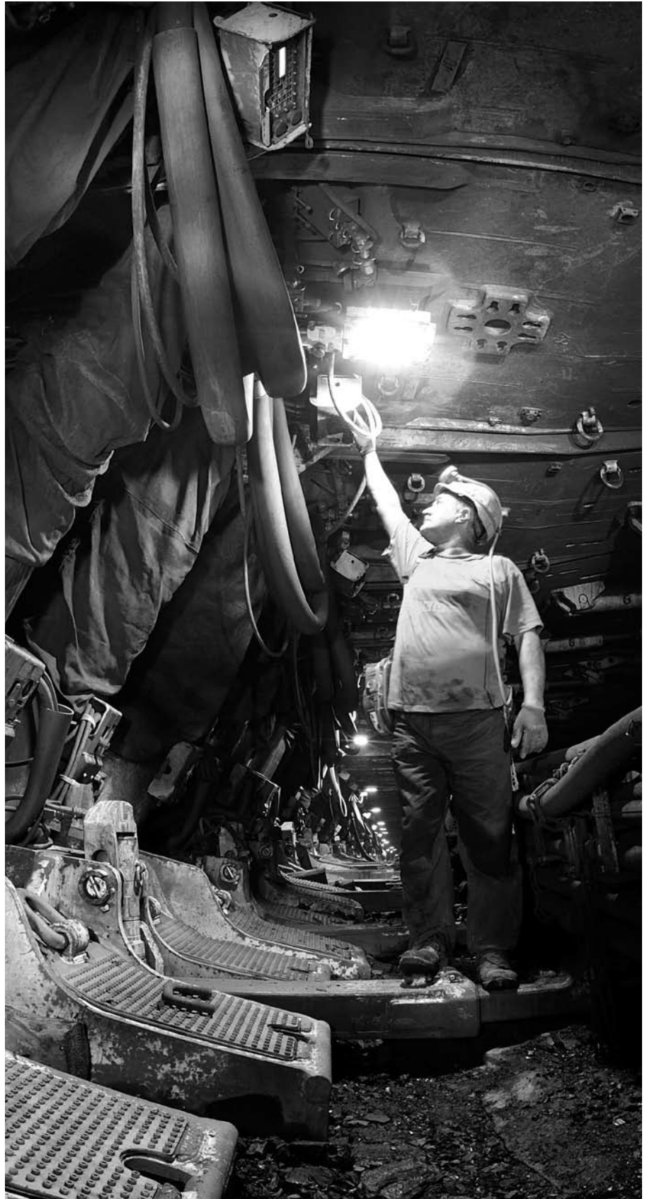
Mid-seam POP 2010 equipment set: shields
