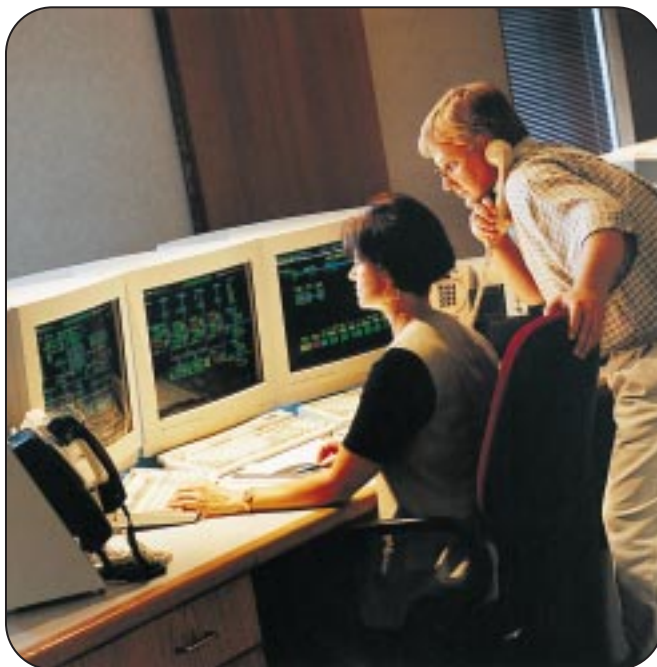
Edmonton Control Centre
