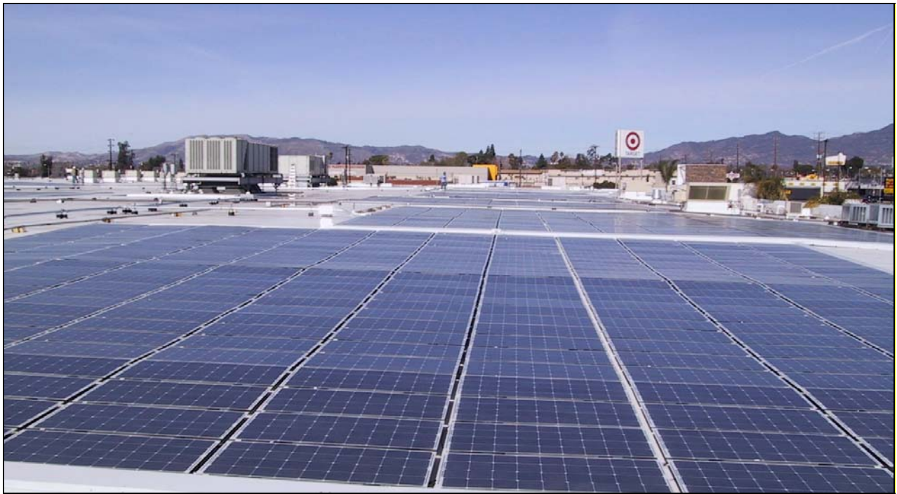
Solar roof panels for harnessing the sun's energy at a Los Angeles Target store
