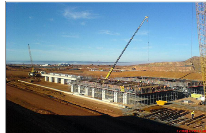
HPGR – Crushing System
