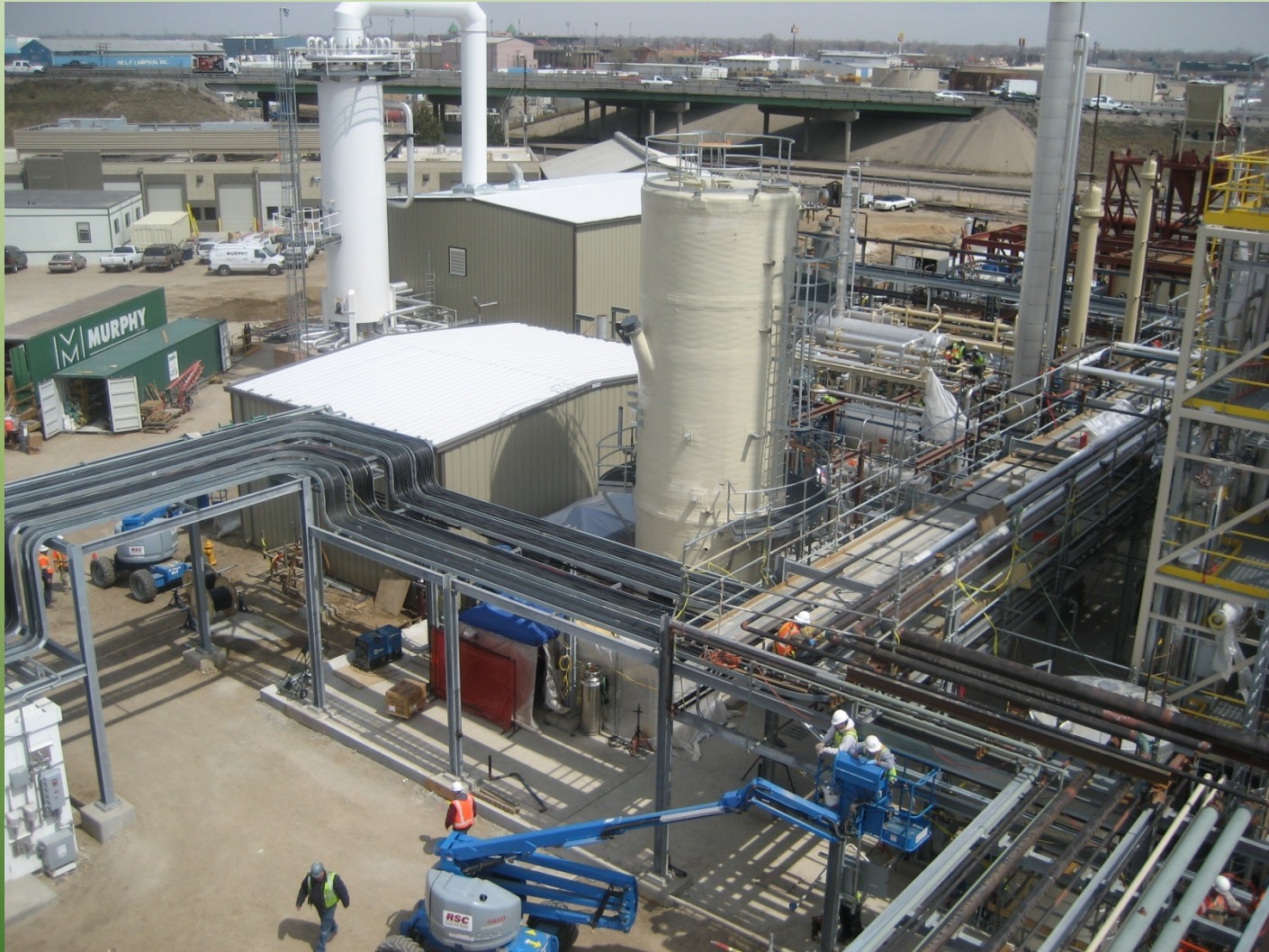
Sulfur building; SMR; main cable tray; main pipe rack; syngas area
