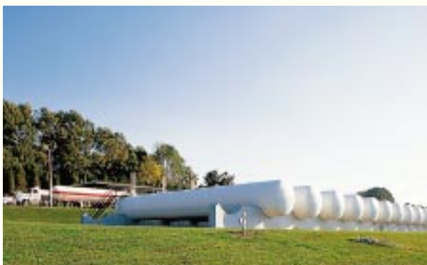
Top: TEPPCO owns approximately 1 million barrels of storage at its Cushing, Okla., terminal. Middle: The Partnership continues to find ways to improve the reliability and integrity of the system, including an ongoing internal inspection program, tank replacements and automation. Bottom: TEPPCO plays a key role in supplying propane for home heating and cooking to rural areas from Arkansas to New England, from facilities like this in Eagle, Pa.
