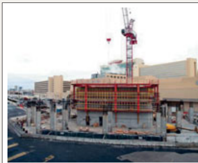
AT THE TAJ MAHAL, CONSTRUCTION OF A $250 MILLION, 40-STORY HOTEL TOWER BEGAN IN JULY 2006 AND IS ON SCHEDULE FOR COMPLETION IN SUMMER 2008. THE NEW HOTEL, DESIGNED TO MAXIMIZE AVAILABLE VIEWS, WILL FEATURE 716 STANDARD GUEST ROOMS AND 70 OCEAN-VIEW SUITES.
