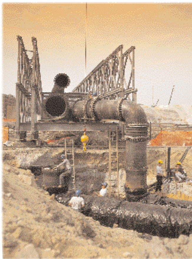
As part of "The Big Dig", a $10 billion public works project targeted for completion in 2004, the city of Boston, Massachusetts utilized U.S. Pipe's broad range of pipe sizes and complementary fittings when relocating a major saltwater cooling system.
