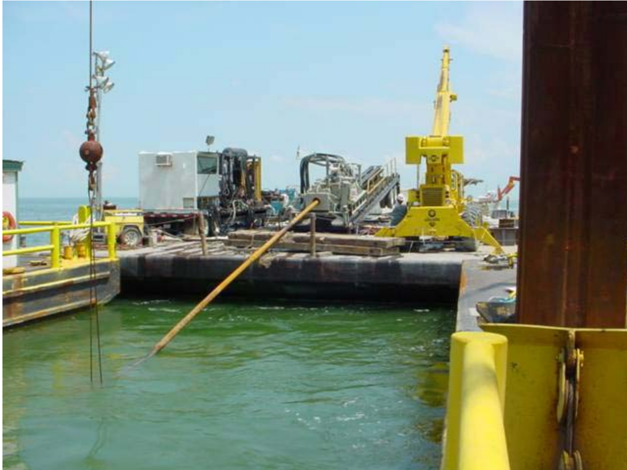
24" Pipeline Horizontal Directional Drill Site on Galveston Bay Water to Water drill under the Texas City Dike & Ship Channel
