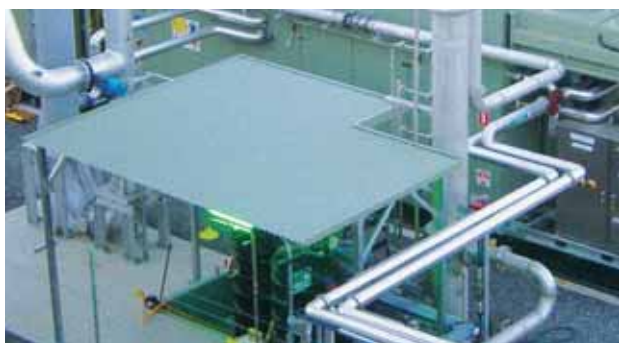
1MW Biogas Cogeneration Facility, Brisbane Water, Qld
