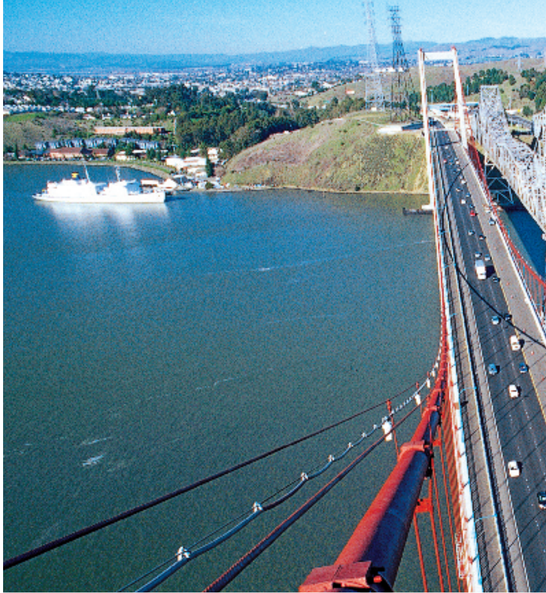
(Right) The Alfred Zampa Memorial Bridge is the first and largest orthotropic box girder suspension bridge in the United States. The bridge spans the Carquinez straits north of San Francisco, California and is protected by Ameron's high-performance coating system.
