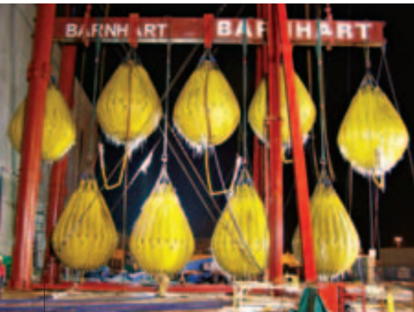
In sub-zero weather, ice forms on the expandable water-filled weights URS used to dead-load test the modular lift tower to ensure its ability to lift the giant MSRs.
