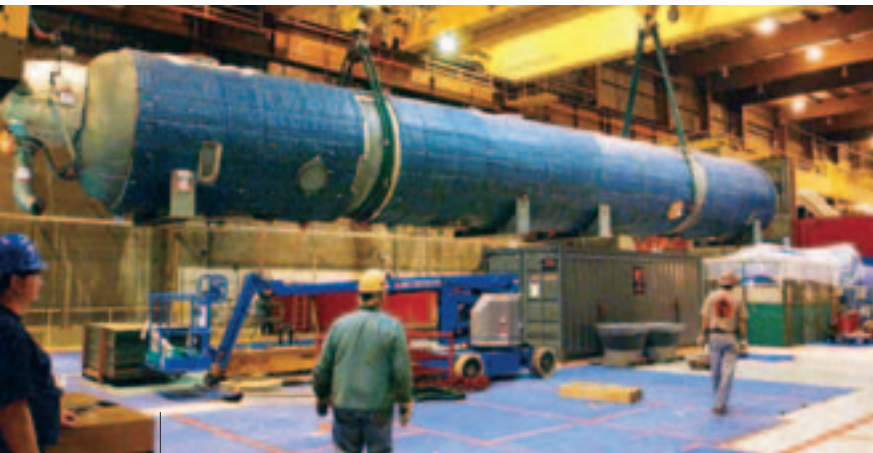
An MSR vessel is carefully transported across the turbine building floor during replacement.
