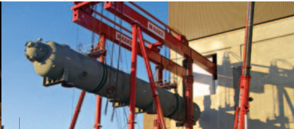
Using the modular lift tower, one of the two new 300-ton MSRs is lifted for installation during URS' retrofit of the plant.
