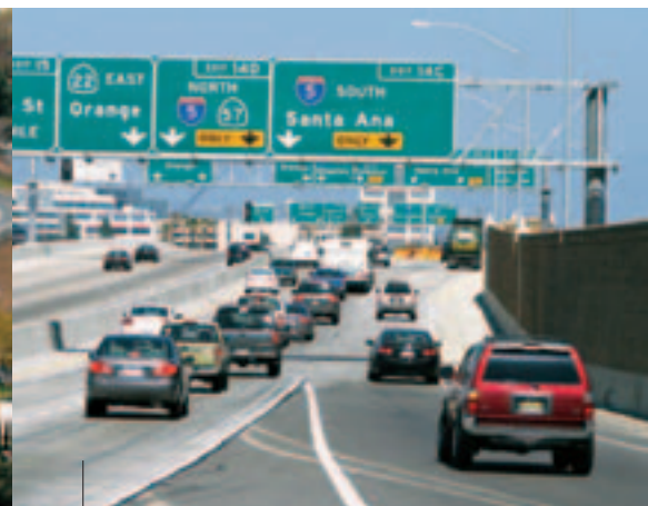
A concrete barrier was added to separate eastbound SR-22 traffic from traffic exiting to southbound Interstate 5.
