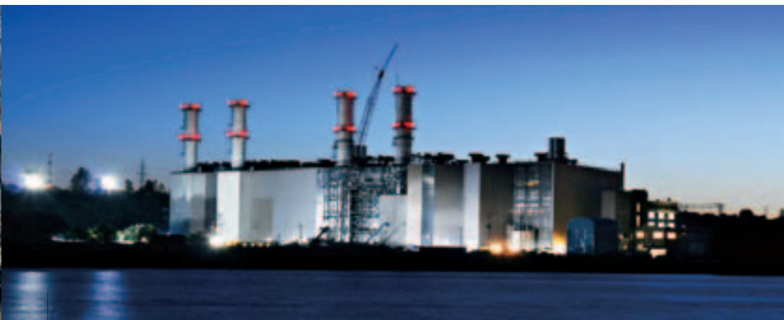
With construction lights facing away from populated areas, Unit 2 rises beside Unit 1.
