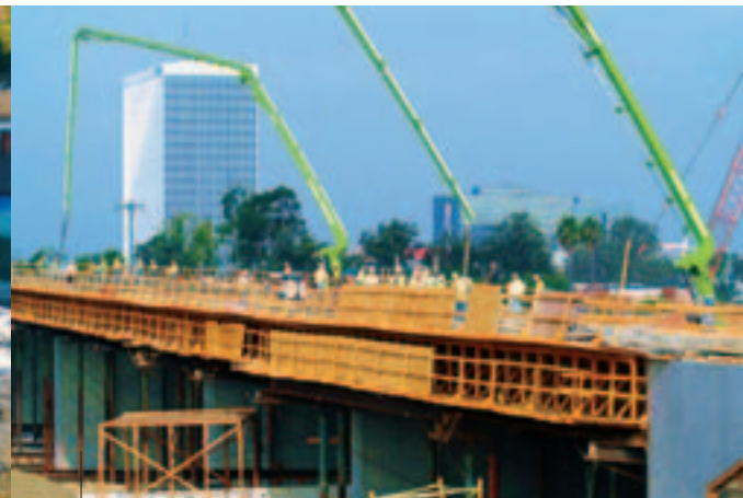
To increase the pace of construction, multiple concrete pumping machines simultaneously placed large quantities of concrete.
