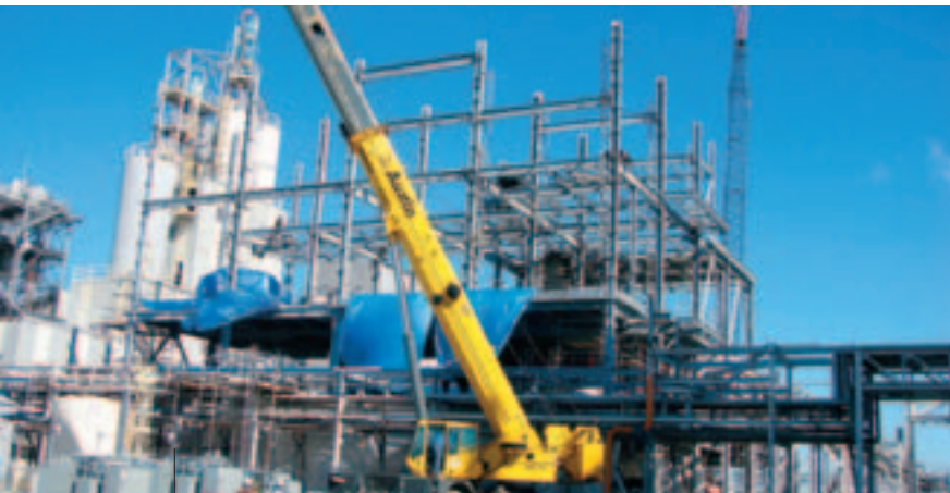
Construction activities included the installation of a new electrical substation that was installed to service the new plant.
