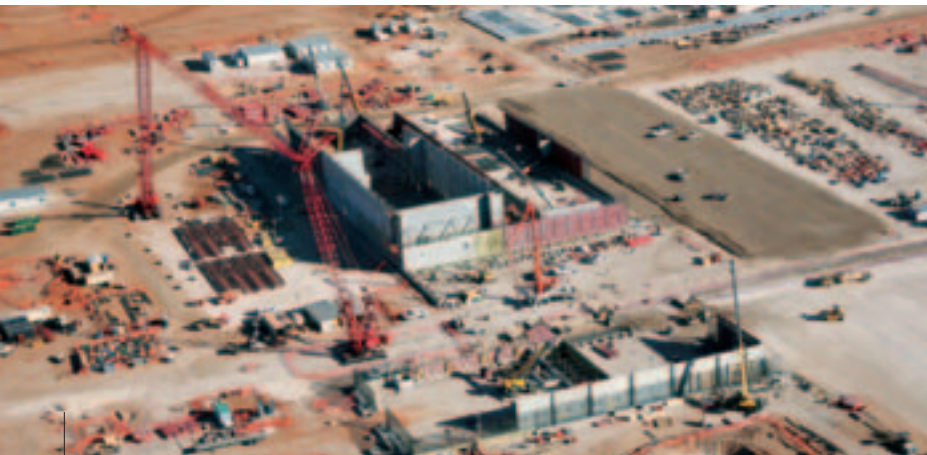
Construction of the National Enrichment Facility is a vital step in the resurgence of the commercial nuclear power industry.
