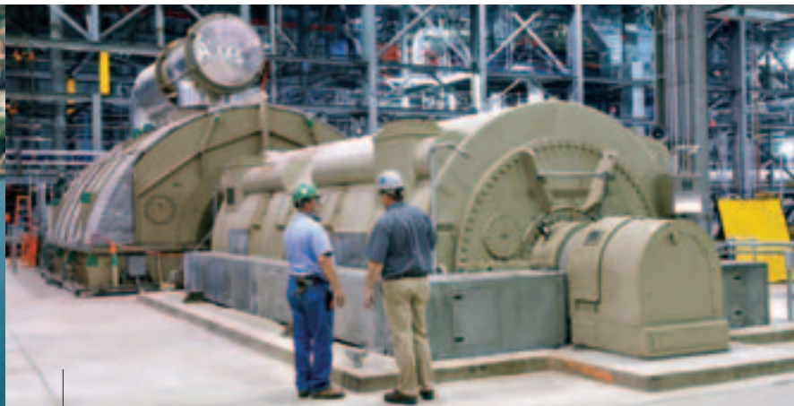
The steam generator is fundamental to the efficiency of the combined-cycle gas-fueled plant.
