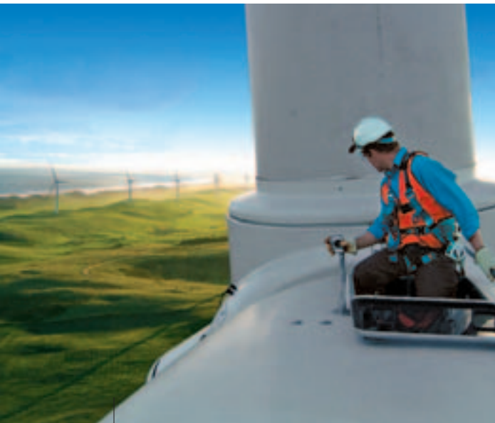
Pacific Hydro, Yambuk Wind Farm, Victoria, Australia
