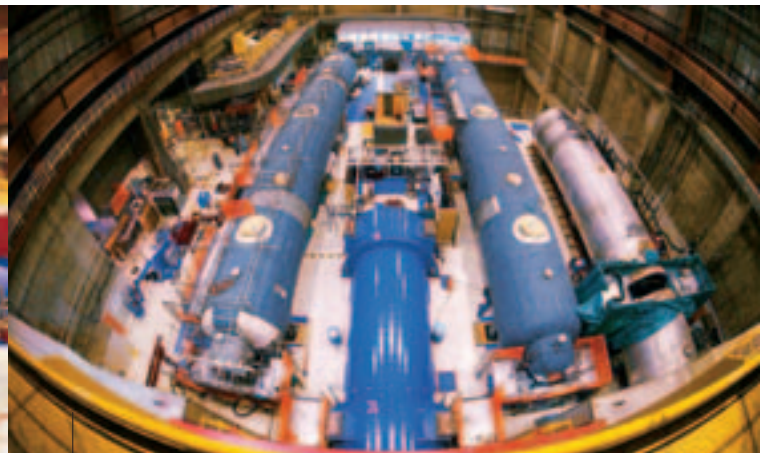
New one-piece MSRs are staged for installation on the turbine deck of the power plant, while one of the old two-piece vessels sits to the right during its removal.
