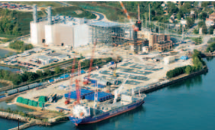
The plant's location on the shores of Lake Michigan enabled URS to have freighters deliver large components directly to the construction site.
