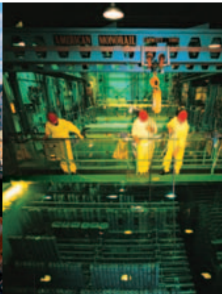
Department of Energy's Savannah River Site, Defense Waste Processing Facility, Aiken, South Carolina
