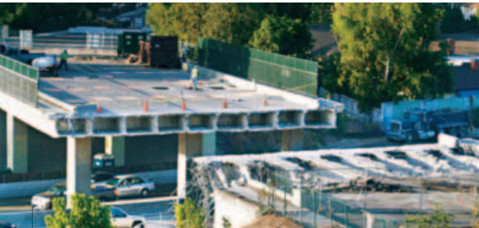
The Lewis Street Bridge over SR-22 was completely demolished and replaced with a new structure.
