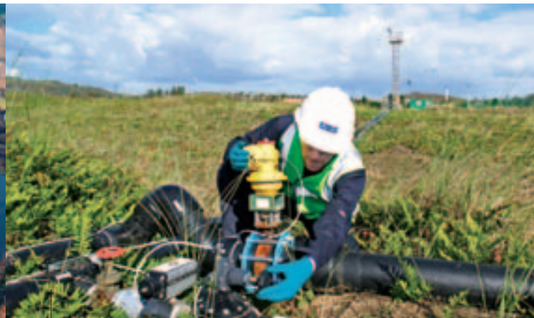
At the Llandarcy site, URS designed and installed a variety of treatment systems to remediate soil and groundwater.
