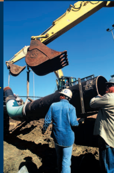
▶ The Explorer Pipeline Mainline Expansion project in the Midwestern United States teamed Willbros Engineers with Willbros RPI.
