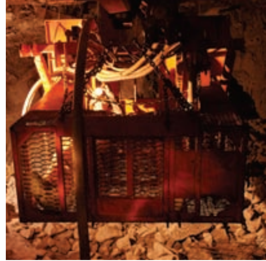
Bottom of the Alimak looking up through flooring mesh as it starts to ascend.
