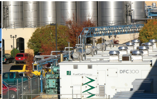
Sierra Nevada Brewing Co., Chico, California Four DFC300A power plants provide one megawatt of 24/7 base load electricity and heat.
