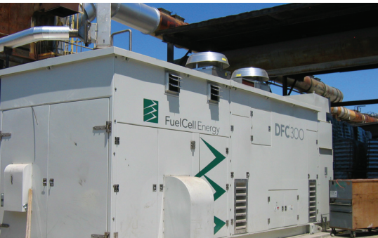
TST, Inc., Fontana, California Two DFC300A power plants provide 500 kilowatts to the aluminum smelter operations.
