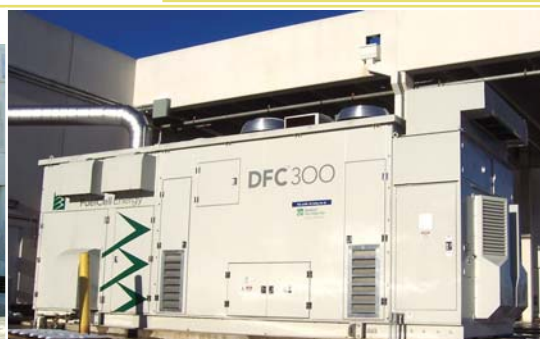
Pepperidge Farm Bakery, Bloomfield, Connecticut Our DFC power plant provides about 20 percent of the facility's base load power, with the heat by-product used for process steam in the bakery.
