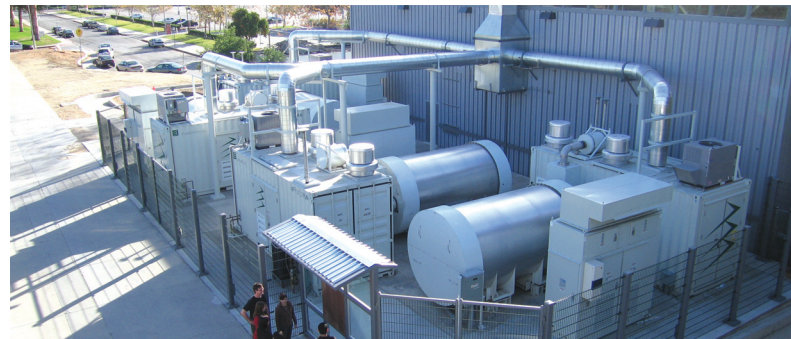
California State University Northridge, Northridge, California Four DFC3000MA power plants located next to CSUN's Student Union Conference and Recreation facilities.
