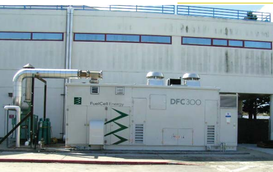
U.S. Postal Service's San Francisco Processing and Distribution Center Our DFC power plant provides part of the base load heat and power requirements.
