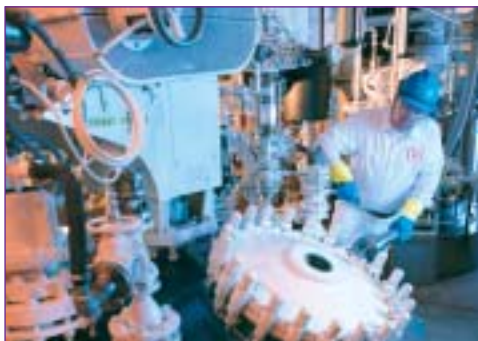
Reactors up to 2,000 gallons at our Sheboygan, Wisconsin plant produce organic chemicals for the Pharmaceutical, agrochemical and material science industries.
