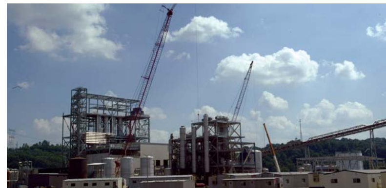
First Bio-Based Materials Plant With joint venture partner Tate & Lyle PLC, we are completing the construction of a new plant in Tennessee that will be used to manufacture Bio-PDO™. This is a key ingredient for our first bio-based polymer, Sorona®. Making Bio-PDO™ from corn uses 40 percent less energy than that needed to produce a petroleum-based equivalent. Our new plant will save the equivalent of 10 million gallons of gasoline per year, or enough to fuel 22,000 cars annually.
