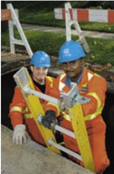
General utility workers John Keenan and Vishnu Gopalsammy working on a gas excavation project; part of the $150 million Con Edison of New York invested in its gas distribution system in 2005.
