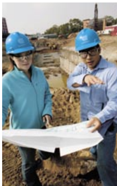
Laura Feeney (l), chief construction inspector, and Brian Yee-Chan (r), chief construction inspector, review plans for the new Mott Haven substation.
