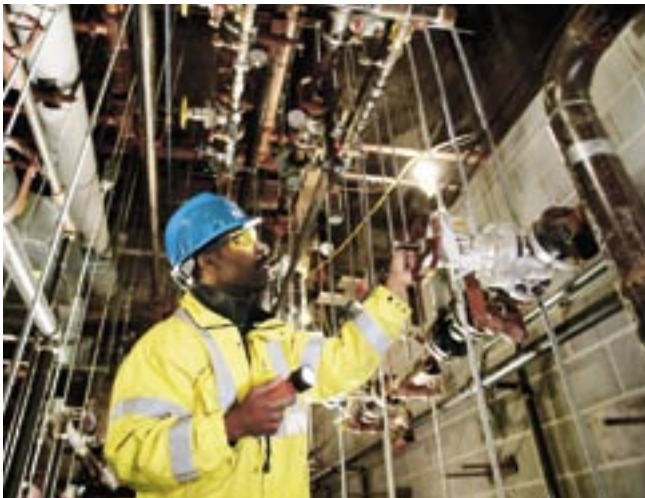
Con Edison's steam system is the largest district steam system in the world. Senior designer Emilio Frederick confirms that the installation matches specifications.
