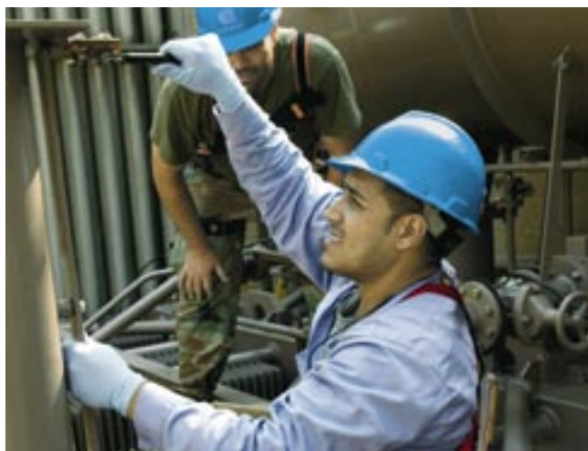
Luis Mendoza III, mechanic A, and Joseph Eckett, mechanic A, connect the fitting on a new transformer.
