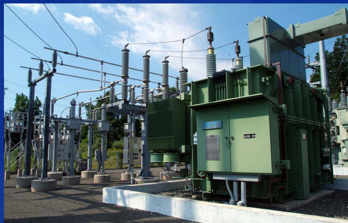
Orangeburg Substation, Orangeburg, NY
