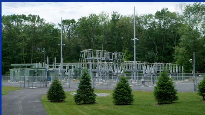
Darlington Substation, Ramsey, NJ
