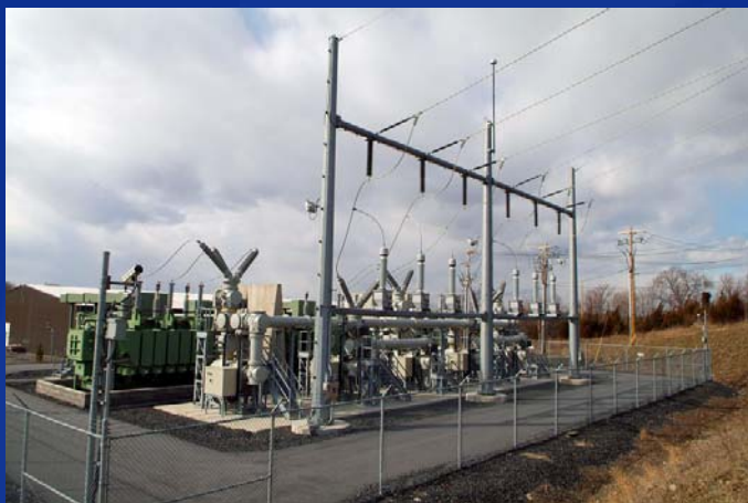
Chester Substation, Chester, NY
