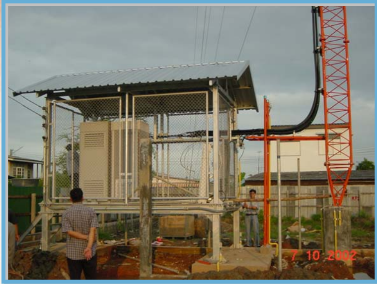
Shelter with fencing: Nokia UltraSite
