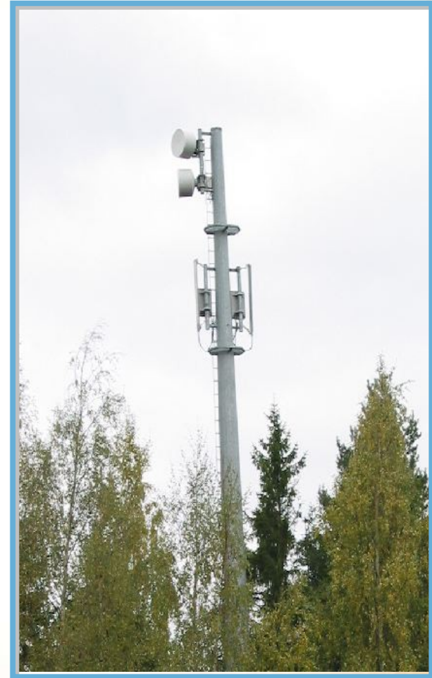
Shelterless site: Nokia MetroSite BTS
